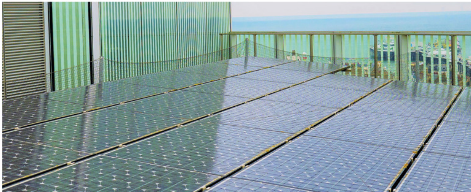
— Solar panels at our UK office.
