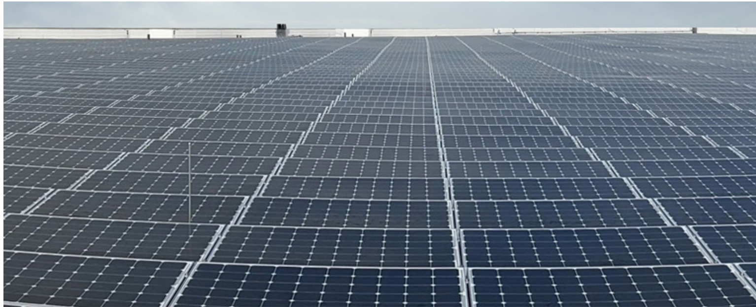
— Solar panels at our North Carolina data center.
